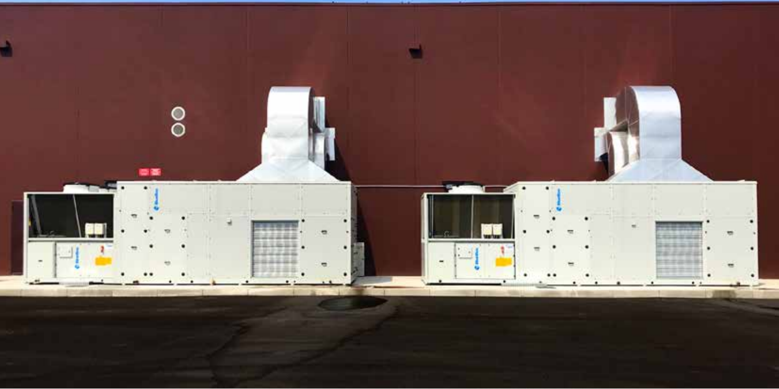
PITTARELLO SHOES, OLBIA Olbia - Italy LAMBDA ECHOS HE HP RS4S SLN supply - 400 kW
