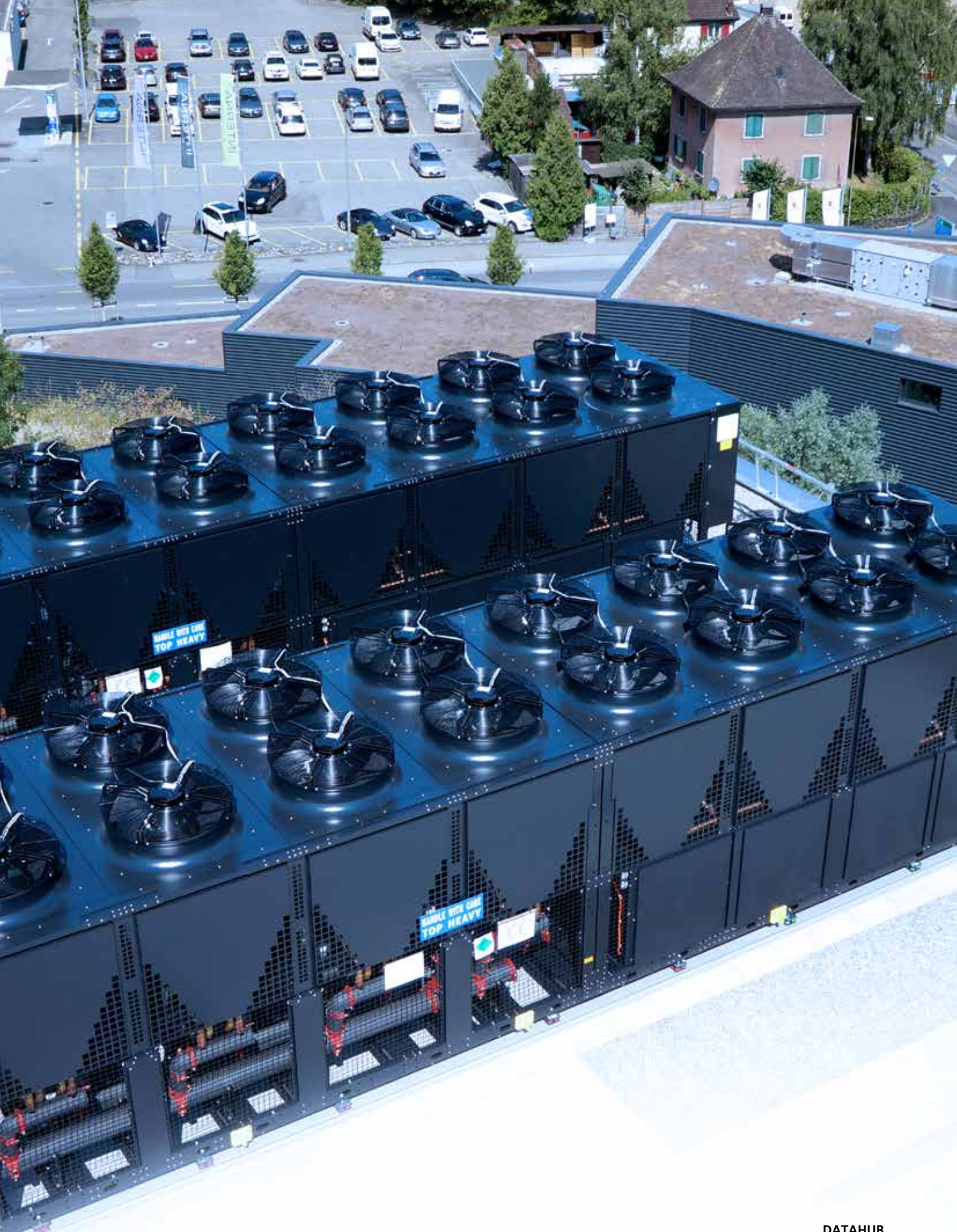
DATAHUB Winterthur - SWITZERLAND 2 x Kappa Rev LGW supply 520 kW
